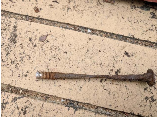
Figure 3 Crevices corrosion in metal bolt embedded in wood
