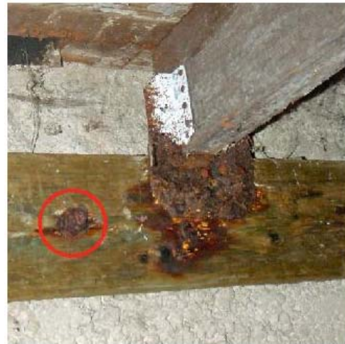
Figure 1 Corrosion of ferrous metal fixture embedded in timber structure [6]
